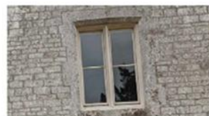
Painted timber frame on sash
