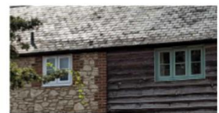
Casement windows (uPvc)
